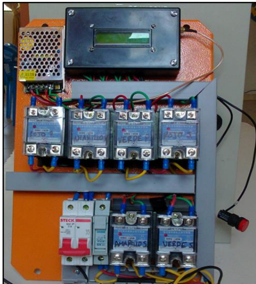
Figure 14. Assembly of the components in metal cabinet
