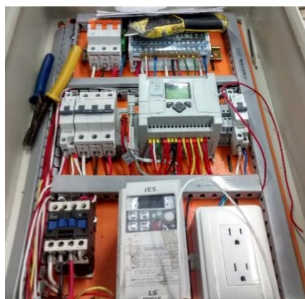
Fig. 5. Tablero de control
