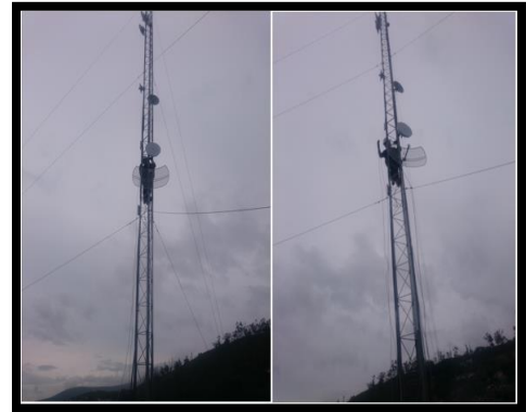
Figure 8. Implementation UTN equipment.
