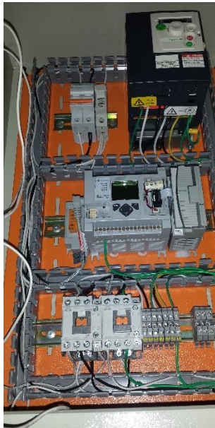
Fig. 6. Wiring the didactic module.
