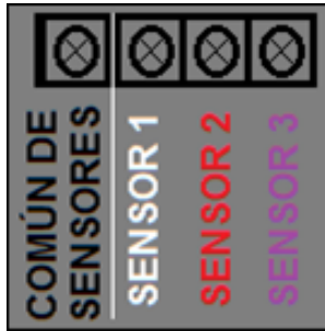
Figure 13. Connection of sensors in the cabinet
