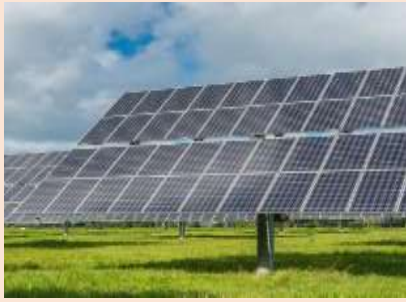
C Solar power
