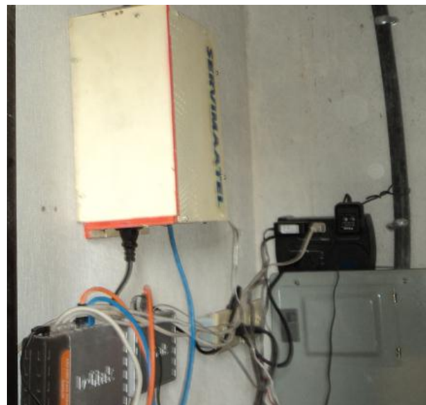
Figure 9. Implementation of central video-telephony in the "LME"
