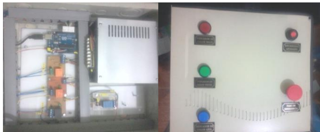
Figure 5. Control Panel Module
