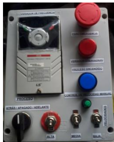
Figura 10: Gabinete de Control
