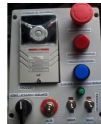
Figure 10: Cabinet de Control
