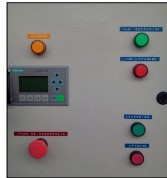
Figure 14. Placement of the buttons and the pilot light on the control panel lights
