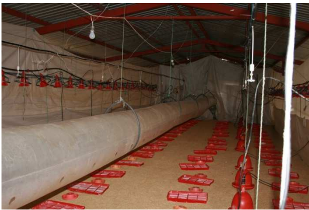
Figure 10.-Heater System in the Barn
