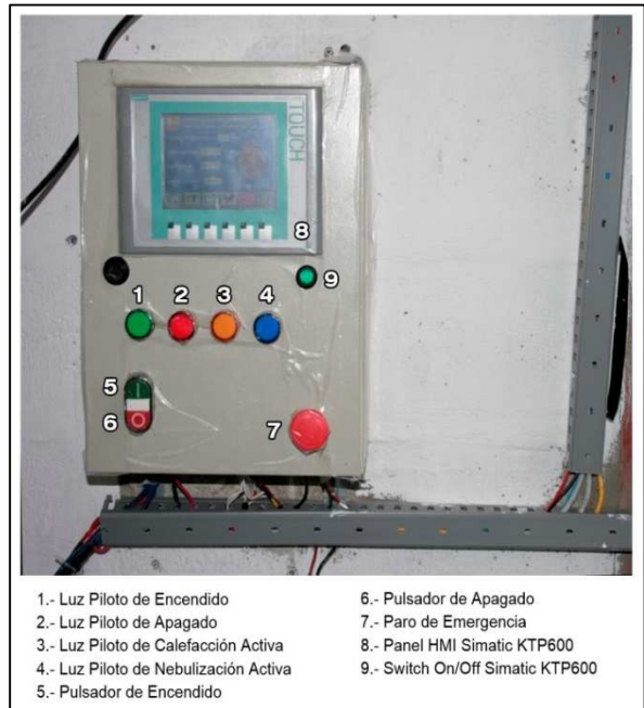
Figure 13.-Control panel- Front View
