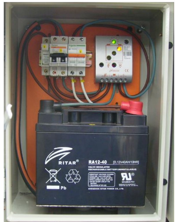
Figure 2 Cabinet of power distribution
