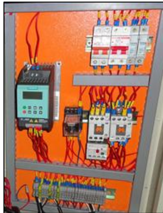
FIGURA III - 7: Tablero de control
