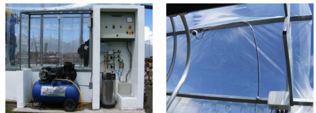
Figure. 7. Pneumatic spraying system
