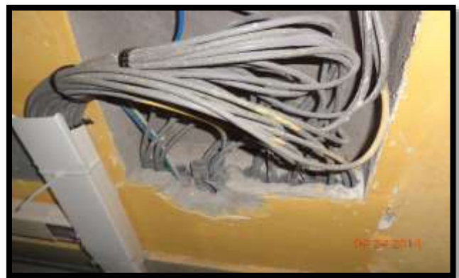
Figure 11. Channelling of cables Picture taken on the premises of the matrix San Antonio by Esmeralda Patiño
