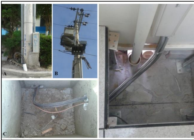
Figure 17. Electric rush CDP Source: Project Design Data Center FICA
