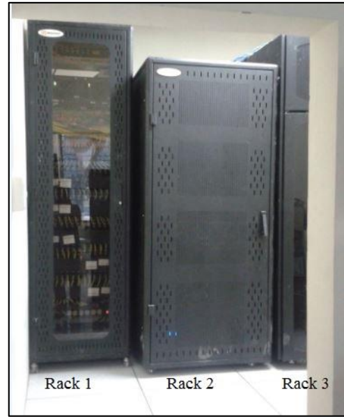
Figura 23. Racks installed in the Data Center Source: Project Design Data Center FICA
