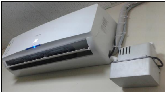
Figura 22. Air Conditioning System installed Source: Project Design Data Center FICA
