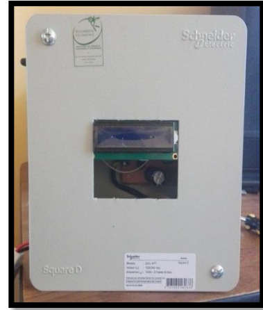
Figure 11. Industrial panel # 1 reception system
