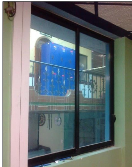
Figure 5: Window inside the Data Center of the COAC Chuchuqui Ltda.
