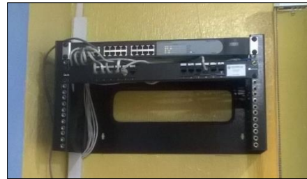
Figure 2: Intermediate connection equipment without protection.
