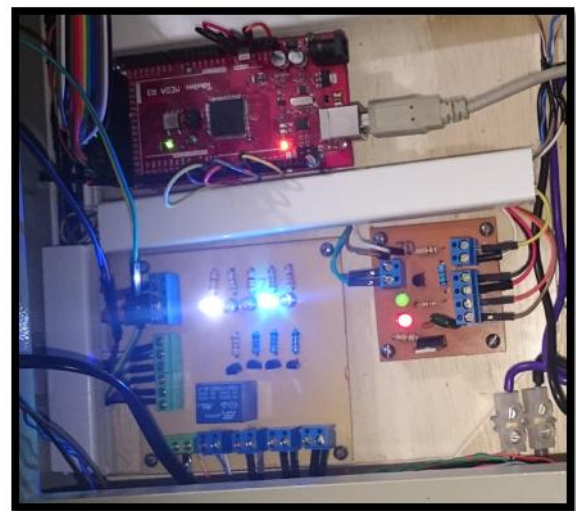
Figure 29 End of process and electric motor activated display Leds
