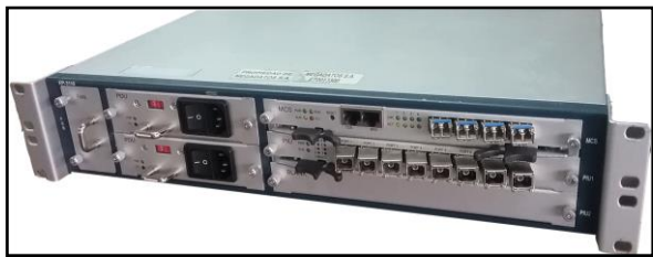
Figure # 6. OLT or optical core team for Gpon network equipment.
