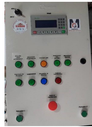
Fig 13 Control Panel Front Panel
