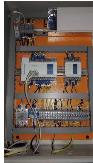
Fig 14 Control panel internal panel
