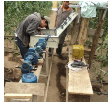
Figure 17 Checking control system uncharged .
