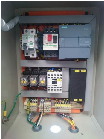
Figure 20: Internal Control Panel view
