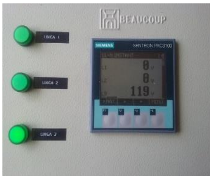
Figure 54. Reading of electrical variables with energy cut
