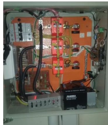
Figure 53. Master node of the system in electrical cabinet
