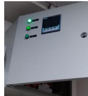
Figure 52. Slave node (PAC3100) in electrical cabinet
