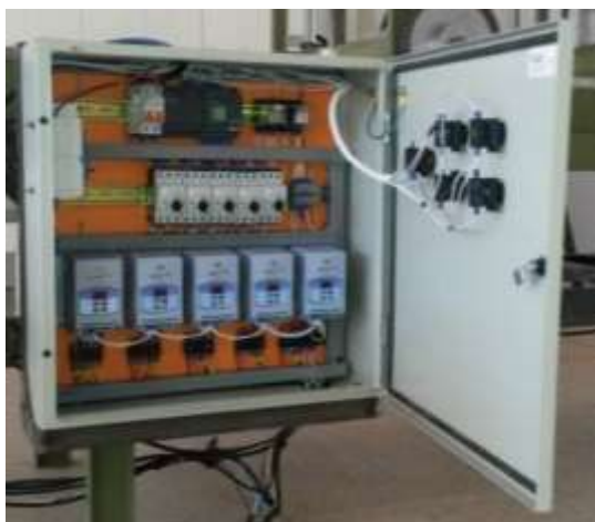
FIGURA 4.19: Tablero de control PLC
