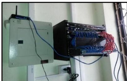
Figure 3. Rack secondary located on the ground floor. Source: GAD Urcuquí.
