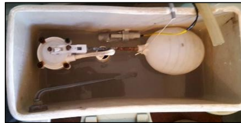
Figure 23. Hose connection with the toilet tank. Source: Authorship
