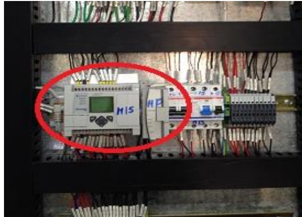
Fig. 35 PLC Allen Bradley MicroLogix 1100
